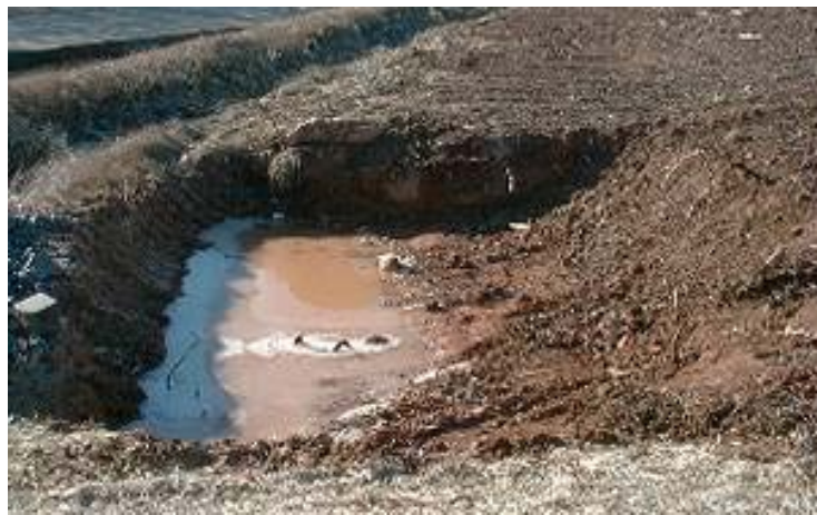
Photograph ST-1. Sediment traps are used to collect sediment-laden runoff from disturbed area. Photo courtesy of EPA Menu of BMPs.
