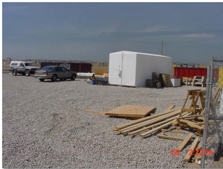
Photograph SSA-1. Example of a staging area with a gravel surface to prevent mud tracking and reduce runoff. Photo courtesy of Douglas County.
