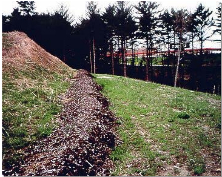
Photograph BB-1. Brush barrier constructed with chipped wood. Photo courtesy of EPA.
